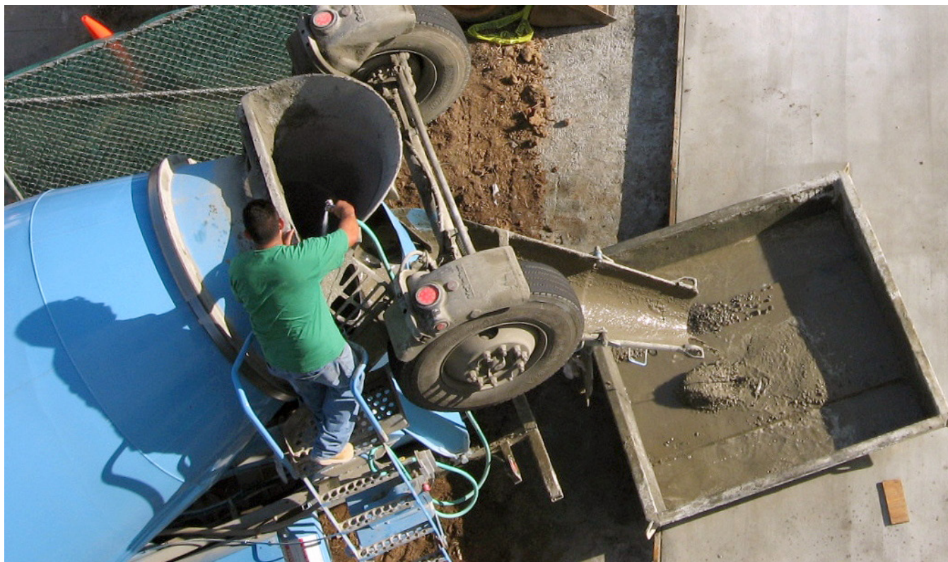
An overhead view of a worker using a concrete mixer to create concrete at a construction site in Los Angeles, California.
