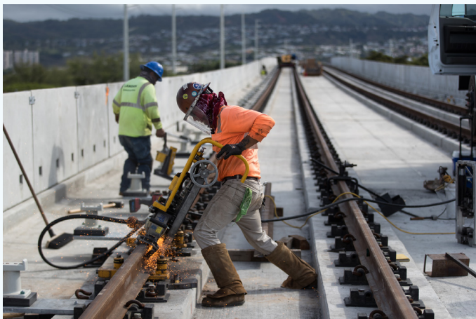
A worker at a construction site for the Honolulu Rail Project in Honolulu, Hawai'i.
